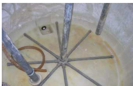
To clean tanks, flush out and then dry to remove final deposits
