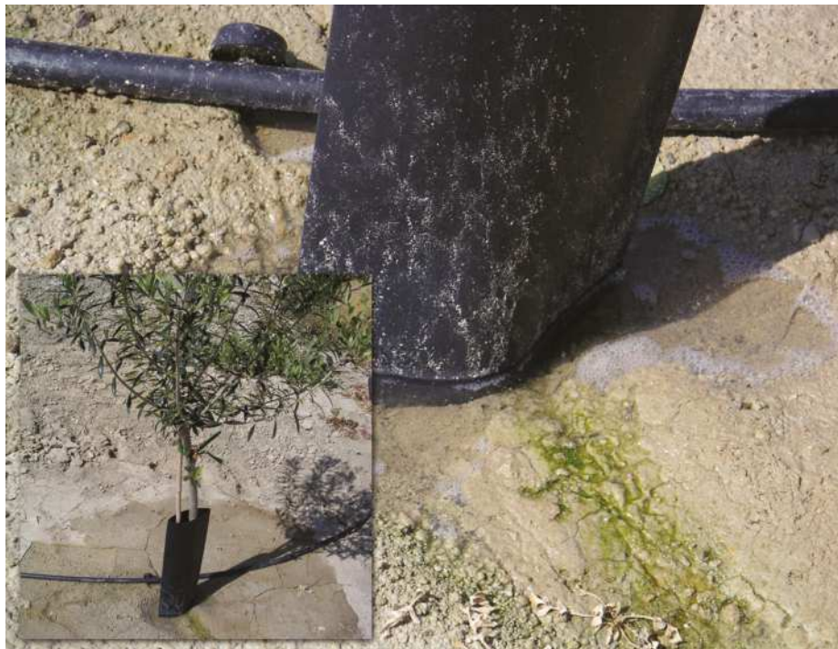
Salinity causes infiltration problems
