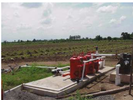
Head unit at pumping station
