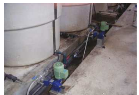
The above photos show head units with two injections
