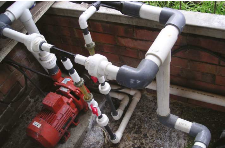
Venturi injection with booster pump
