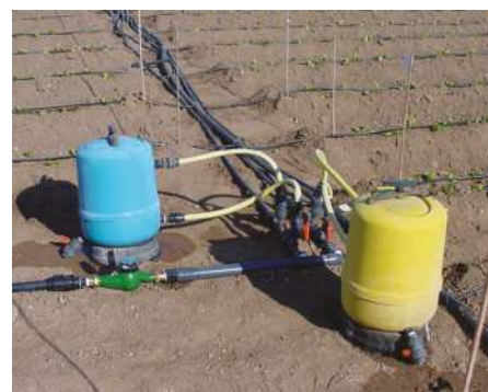
By-pass pressure tank
