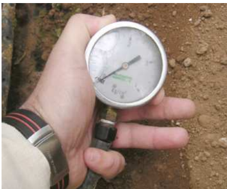
Pressure Gauge for monitoring pressure in different parts of the system
