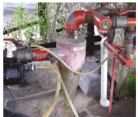
Head unit maintenance is essential
