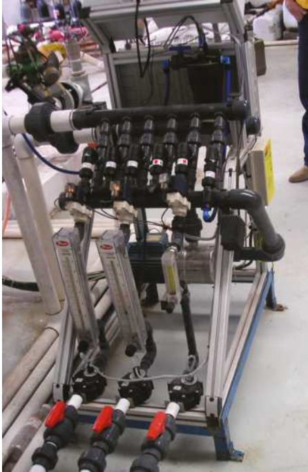
Automated system with a number of injectors
