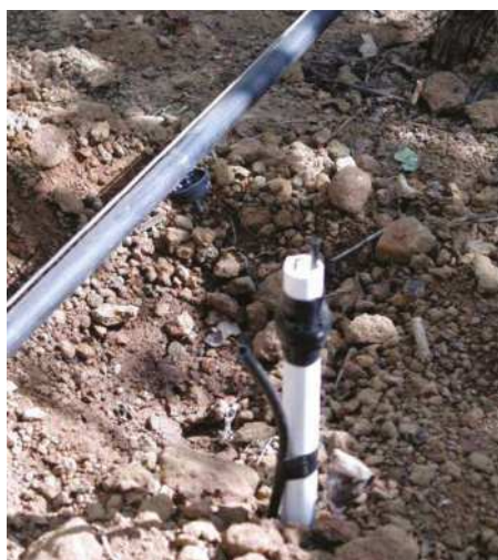
The photos above show the funnel system for collecting soil solutions in South Africa
